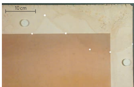
Fig. 3: Water and mould stains after washing.
