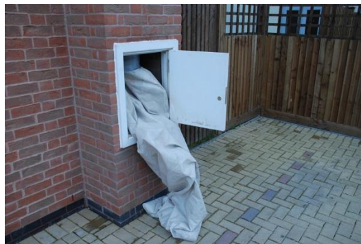
Vent Sock connection
