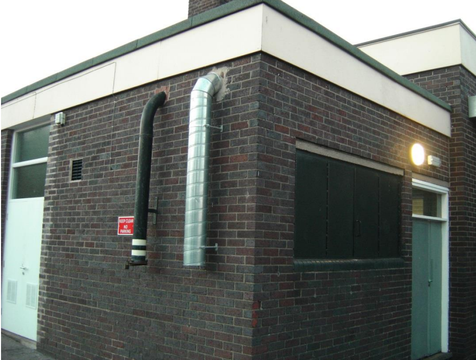
Externally located Pellet Delivery Pipe (black pipe on LHS) and Air Vent Pipe (Silver Spiral Steel on RHS). System Size: Herz Firematic 90Kw.
